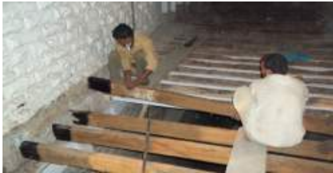
The fixing of the rafters with its edges coated in Black Japan.
