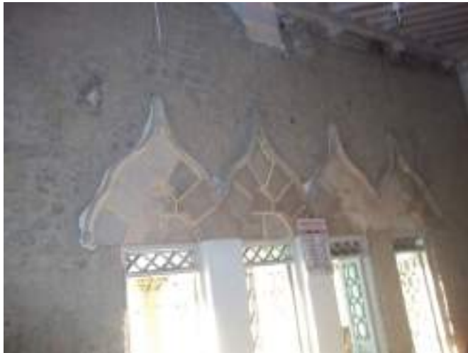
A damaged portion of interior wall.
