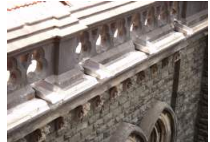
The additional water spouts.
