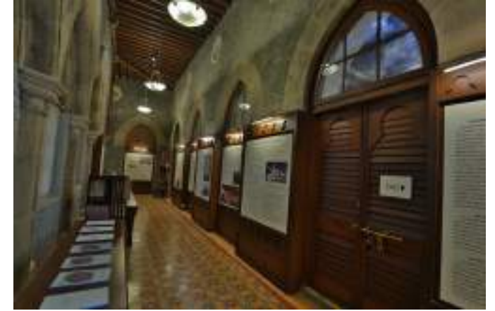
A view of the door restoration, flooring, ceiling rafters and complete civil restoration works of the museum.
