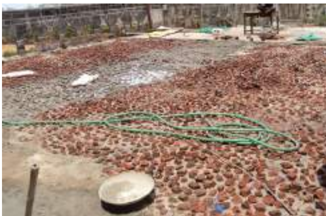
Images showing the stages of structural consolidation and terrace water proofing of the flat roof facing the Oval Maidaan.
